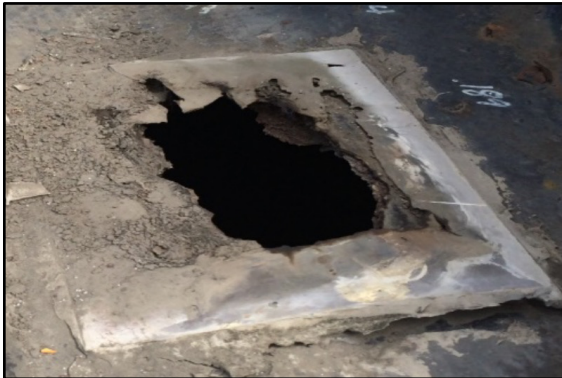
Before: Damaged tank roof.
